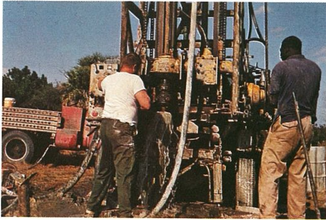
Observation well construction at Lands End; photo by D. Duncan, S. C. Water Resources Commission.
